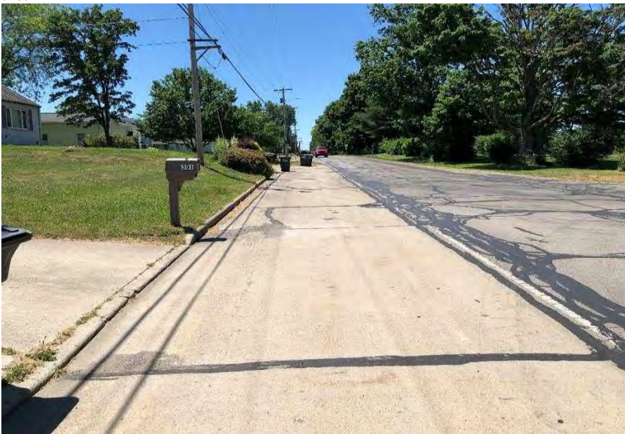
Photo 70. Facing west along southside of Drake Rd from eastern terminus of the investigated area.
