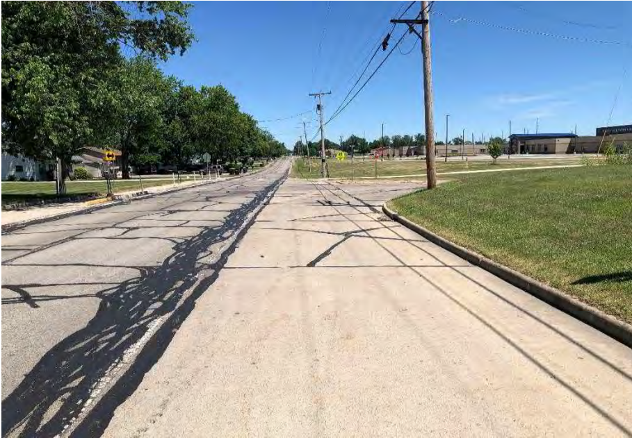
Photo 69. Facing east along southside of Drake Rd from eastern terminus of the investigated area.
