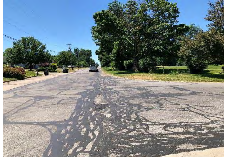
Photo 68. Facing west along northside of Drake Rd from eastern terminus of the investigated area.
